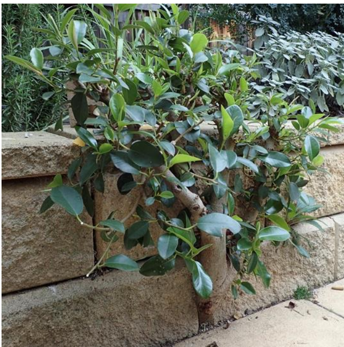
Growing in the cracks
